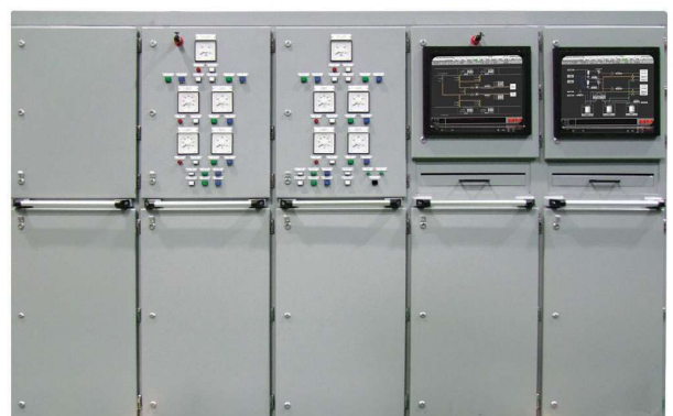
● Fuel Cell Control Board (FCCB)
