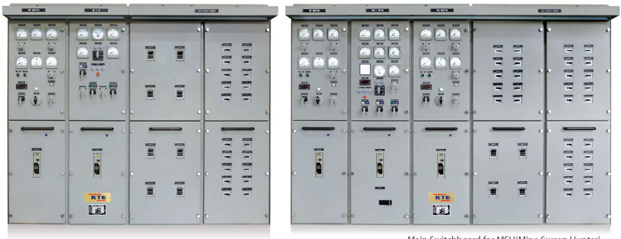
Main Switchboard for MSH(Mine Sweep Hunter)
